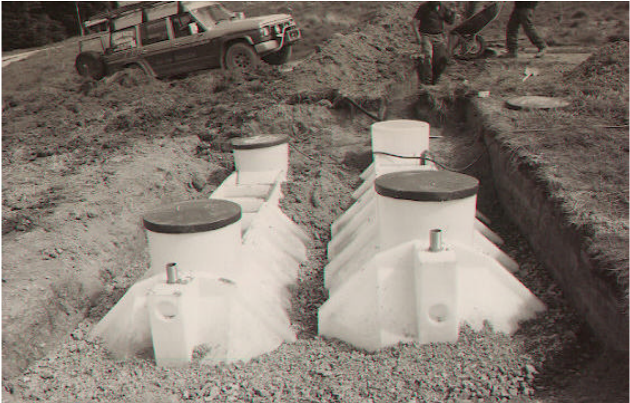
Figure 3. Solwind Dual Chamber Polyethylene Digester System Shown “in-ground” [SOL-W].
